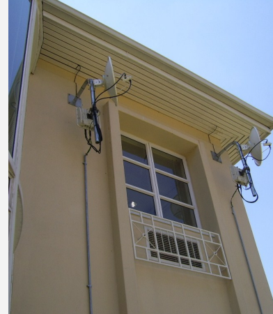
Installation at Bryanston Head Office
