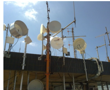
Typical High Site installation
