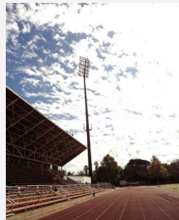
Ikageng stadium floodlight repeater
