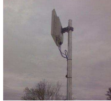
Comsol ~ Motorola: Wireless Ethernet Bridges used to link main facilities Durban to Pietermaritzburg and MTB Durban to Westville admin
