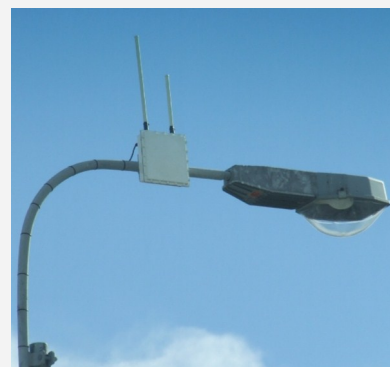
Access point mounted on streetlight
